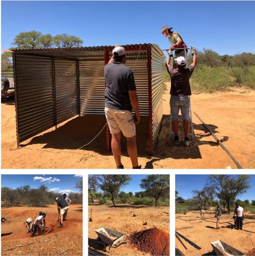
Figures 3 to49: The construction of the corrugated houses for Anaki and the family of the late Chief Sangiro gets underway
